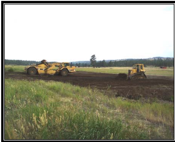
Phase 2 McCoy Creek channel construction. Photo illustrates use of large construction equipment including scraper loaders and track-mounted dozers.
