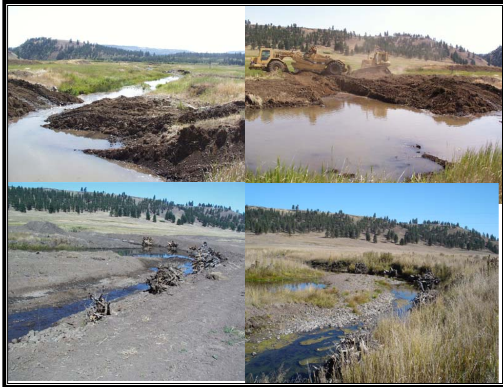
Photo sequence taken illustrates lower channel diversion in phase 3 project reach. Upper photos show initial channel diversion efforts. Lower photos show the constructed outside meander with rootwad revetments and revegetation activities. Note vegetative recovery in lower right photo following installation of shrubs and sedge/rush mats.
