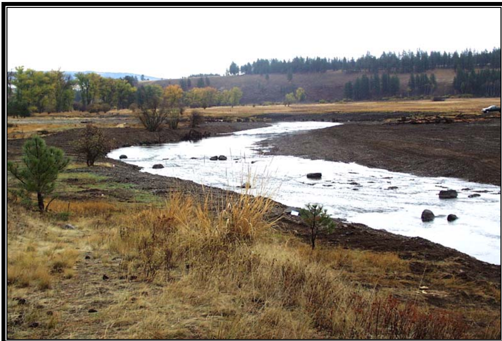
Mainstem Grande Ronde Project – photo illustrates post construction of new meander channel just upstream of Bear Creek. Channel diversion is complete and revegetation activities have been initiated.
