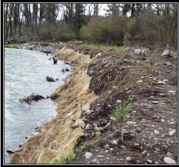
Mainstem GR Phase I Photo Point (Oct 99'). Streambank stabilization using rootwad revetments and bioengineering to meet landowner streambank stabilization objectives.
