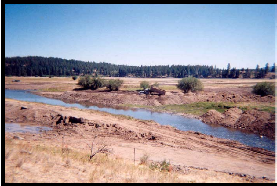
Mainstem Grande Ronde Project – photo shows the construction of a pointbar along the right bank. Material was sorted and transported from the new channel to the pointbar by truck in order to avoid sedimentation. A dozer was later used to shape the pointbar surface.
