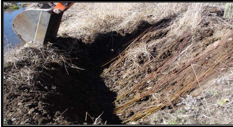
Mainstem Grande Ronde River – Shrub planting included mechanical installation of bundled, conditioned live willow whips. Strategy includes deep installation of material near water sources to facilitate recovery.
