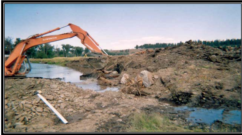
Mainstem Grande Ronde Project – photo shows the construction of a rootwad revetment along the right bank at site 4, just downstream of Bear Creek. Rootwads with 20-foot boles are placed on top of footer logs and then backfilled. The upper portion of the bank will be tapered back to a 4:1 slope.
