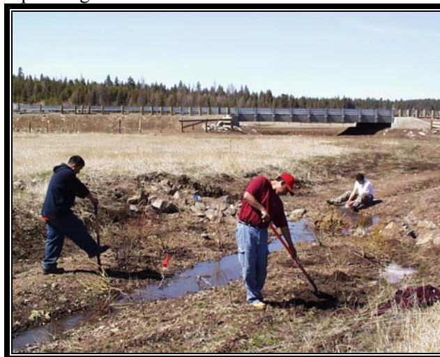
Salmon Corps planting vegetation on the McCoy Creek Restoration channel following construction.
