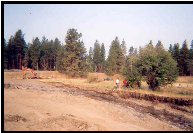
Mainstem Grande Ronde Project – photo of new meander channel looking upstream. Grande Ronde River channel is located to the left of photo. The excavator is shaping the left bank.
