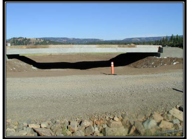
New McCoy Creek bridge provides greater capacity to better provide floodplain connectivity.
