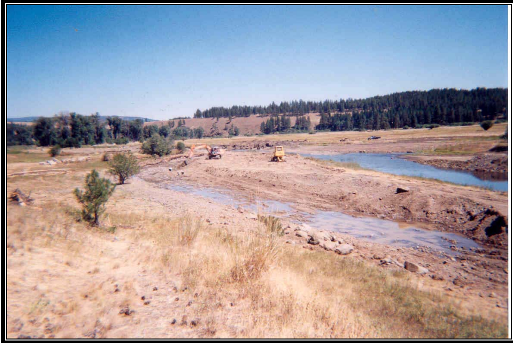
Mainstem Grande Ronde Project – photo illustrates the construction of new meander channel just upstream of Bear Creek. The excavator is shaping the bankfull channel form and right bank. In this photo the Grande Ronde River is still flowing in its old location along the right side.
