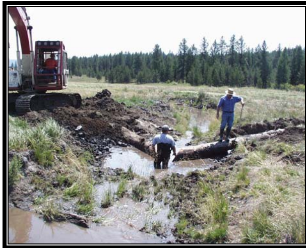
Installation of log "V" weir for streambed grade control and stream gaging station
