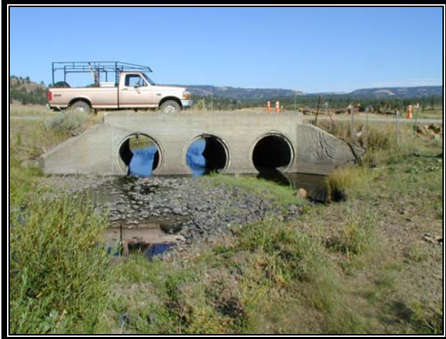
Pre-project triple culvert on McIntyre Road. Existing structure was severely undersized for McCoy Creek.
